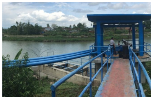
Figure 4. Transmission Pipe in Intake 2
